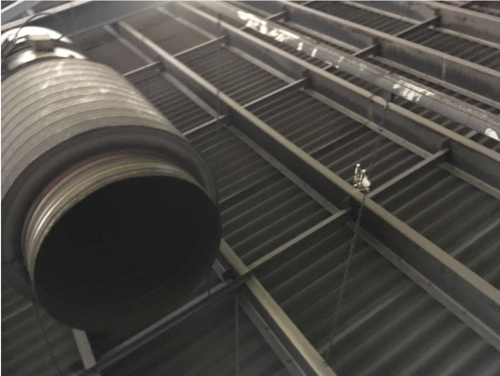
Figure 1 Location of samplers besides vents inside furnace house at site USI-2.
